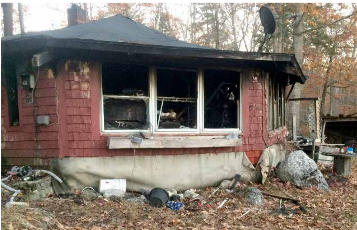
The Mandala house after the fire. The fire burned extremely hot and very little of the structure was left in the end
